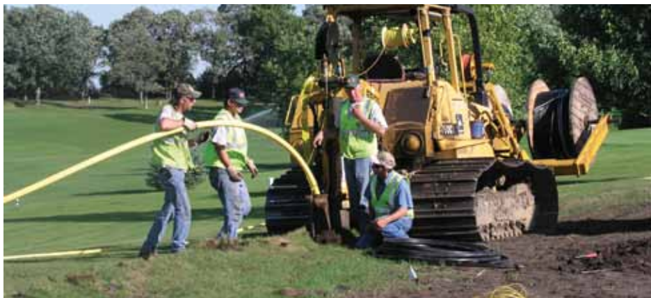
Employees of ACS Construction Services work on installation of a gas line in Perham
